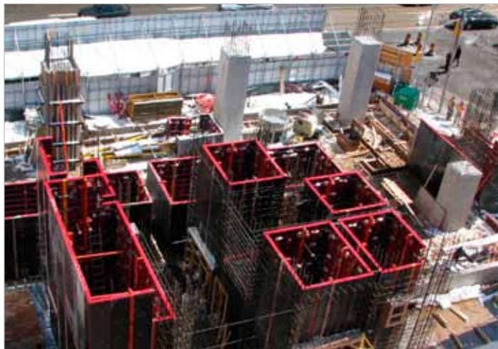
Big Project. When completed in 2013, the SickKids Research and Learning Tower will be a 750,000 square-foot facility with 21 stories, and three levels of underground parking. The project is designed to achieve LEED® Gold Certification for sustainable design.
