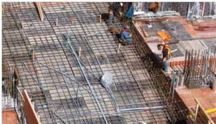
At the jobsite. C&T Reinforcing Steel has been serving customers since 1965. The Toronto-based company uses aSa Computer Shearing to plan fabrication, reduce scrap, and improve productivity.
