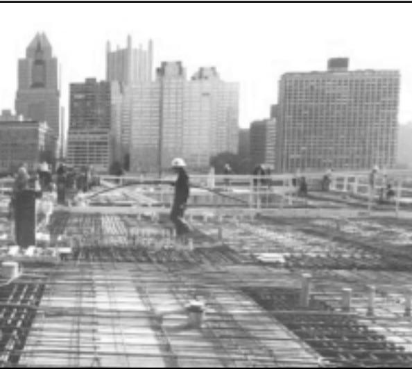
Zottola-Simpson Rebar used aSa software to help detail, fabricate, and deliver 3,800 tons of reinforcing for the Pirates' PNC Park.
