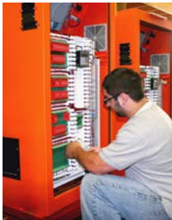
Inside the box. A.J. Guarino wiring an Opto-Shear for a new customer.
